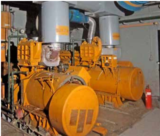
Generators. Photo Tim Wellburn
